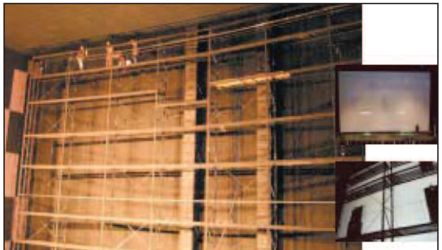
MEGAsystems installation, Memphis, Tennessee and Chorpus Christi, Texas.
